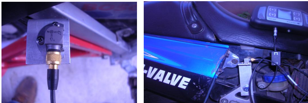
Figure 7: Triaxial accelerometer and vibration analyzer
