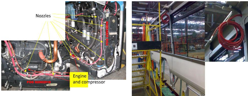
Figure 7. Nozzles of the fire-extinguishing system, positioned in the engine compartment
